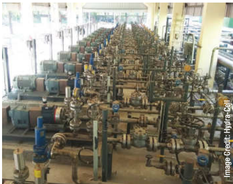
Testing investigated how to minimise shear effects during polymer flooding.
