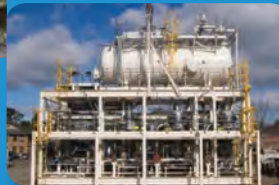
Produced Water Treatment
