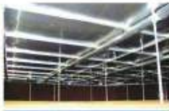
Internal floating roofs
