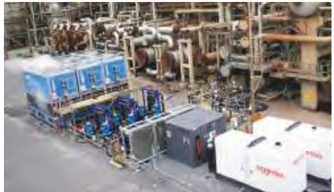
Aggreko cooling towers can help operators to maintain or increase productivity during the summer months
