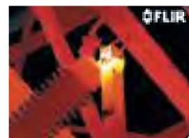
Bad high voltage connection
